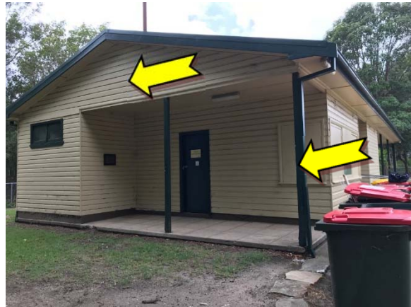
Photo 10. Exterior, throughout, walls and features – suspected lead-containing cream and green upper coloured paint systems.
