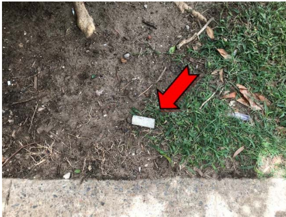
Photo 3. Exterior, throughout, ground – asbestos-containing fibre cement debris.
