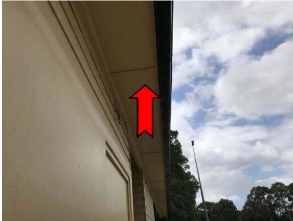
Photo 1. Exterior, throughout, eaves – asbestos-containing fibre cement sheeting.
