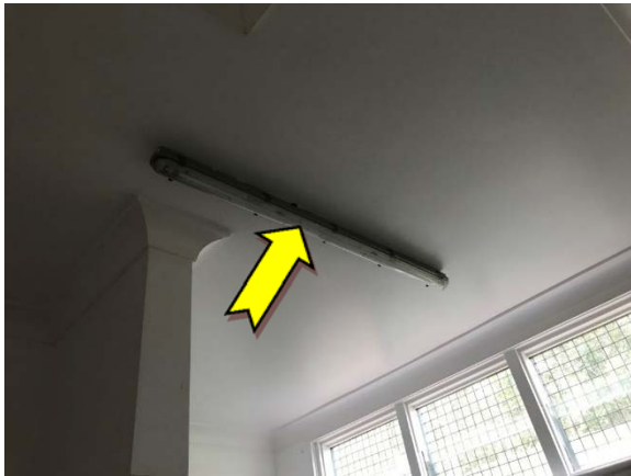
Photo 9. Interior, throughout, single tube fluorescent light fitting – suspected PCB-containing capacitors.
