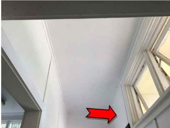
Photo 7. Interior, men's toilet lobby, high level infill panel – assumed asbestos-containing fibre cement sheeting.
