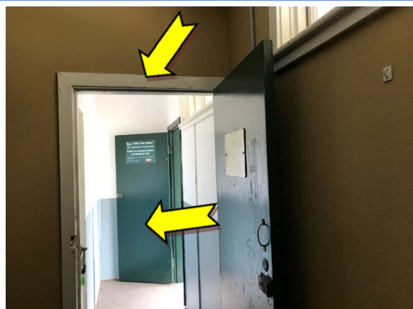
Photo 12. Interior, throughout, door frames and doors – suspected lead-containing white and green upper coloured paint systems.
